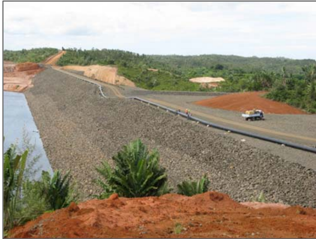
Figure 2. A 2-Year Starter Dam for a 30-year Mine Tailing Facility in Africa, as an Illustration of a Tailings Facility.
